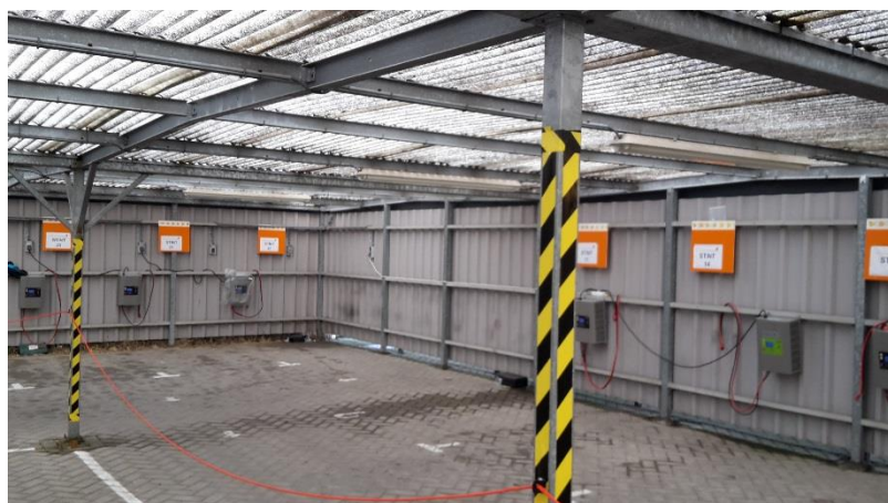
Figure 7. PostNL vehicle charging stations.
